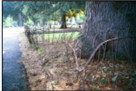
This wire fence has been damaged beyond repair. Replacement with a similar fence is recommended.
